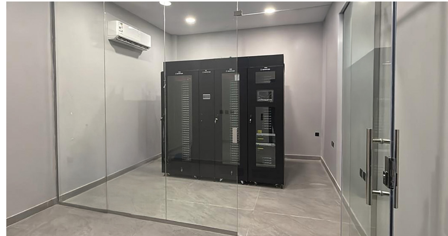
Smart Modular Data Centre solution at Al-Rawaf's headquarters
