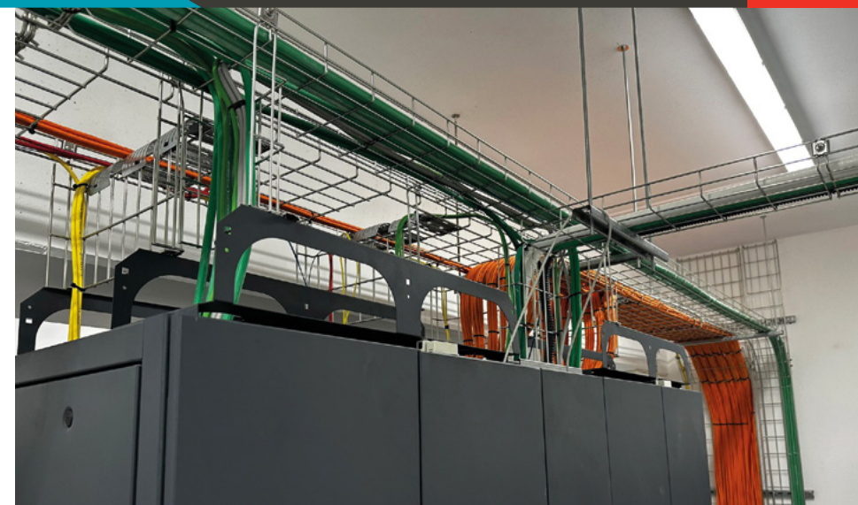
The Smart Modular Data Centre (SMDC) is the central node of structured cabling.
