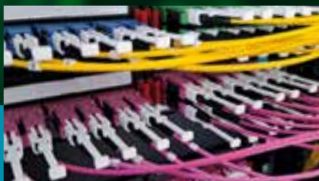
MEDIUM-DENSITY DATA CENTRE SOLUTION (MD-DCS)
