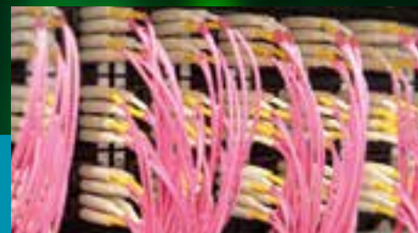
FIBRE OPTIC DATA CENTRE SOLUTION (FO-DCS)
