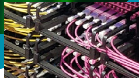
HIGH-DENSITY DATA CENTRE SOLUTION (HD-DCS)
