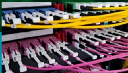
MEDIUM-DENSITY DATA CENTRE SOLUTION (MD-DCS)
